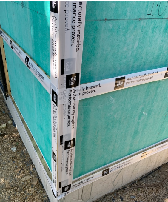
FIGURE 3. BARRIER TAPE STAPLED TO H3 TIMBER CAVITY BATTEN
